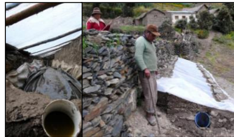
PLASTIC BIOGAS PLANT WITH SOLAR CANOPY
